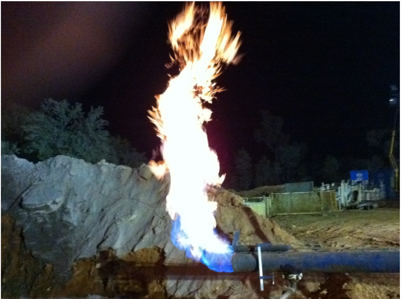
Picture of gas burning from the end of the 8" diameter blooie pipeline, venting Armour Energy's Cow Lagoon 1 well
